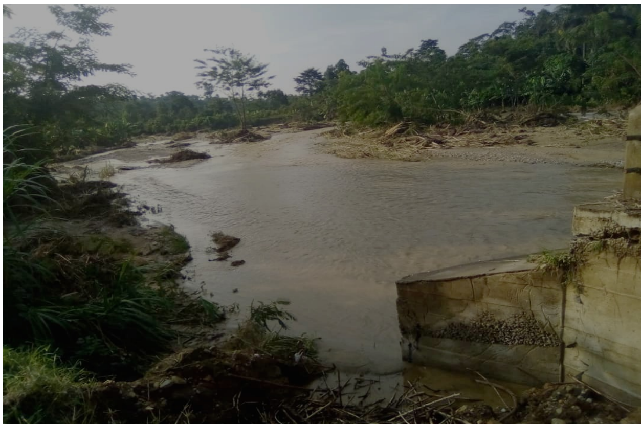
Figure 6: Broken Bridge due to flooding on River Lugo that originates from Rwenzori National Park and drains Semiliki River through Semiliki National Park–Kisuba Sub-county –Bundibugyo District
